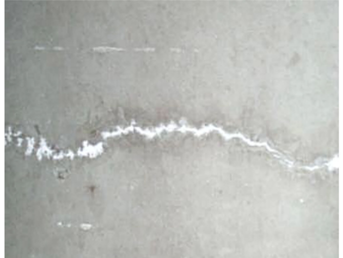
FIG. 3 Calcium Carbonate Filled Crack
